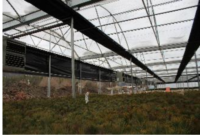
Figure 6.3 A double-layer polyethylene gutter-connected greenhouse designed to grow tree seedlings in California. Note the roll-up walls and the black-cloth system for dormancy induction using shortened photoperiod. There are also lights to extend the photo period.
