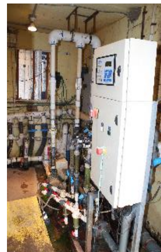
Figure 6.4 Irrigation pumps and fertilizer injector.
